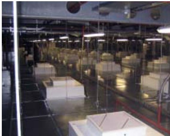
Infusion therapy goods are manufactured under stringent FDA regulations in new clean rooms
